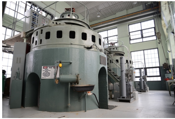
Figure 5-5. Fairfax Falls Hydro Turbine Generators
